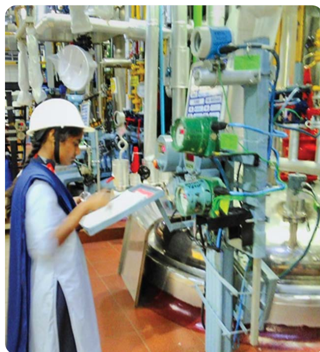
■ Sangini working at PPL Plant, Digwal
