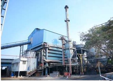
16 TPH Solid Fuel Boiler
